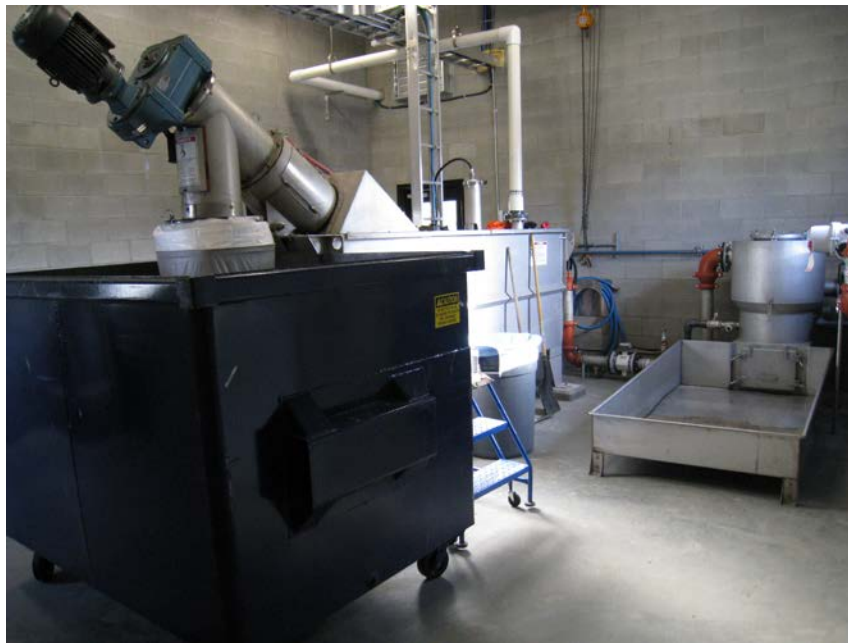
Figure 10 – Septage Receiving Facility
