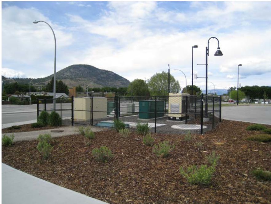
Figure 3 – SOEC Lift Station
