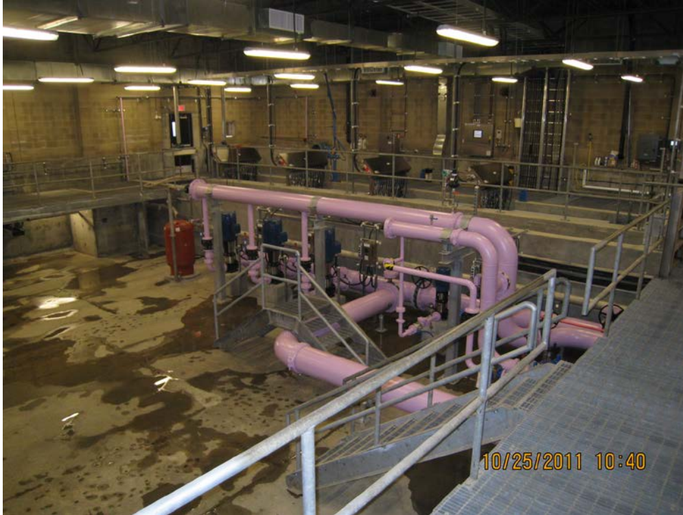
Figure 6 – Reclaimed Water Pumping System and UV Disinfection
