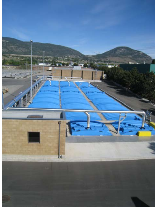
Figure 7 – Primary Clarifier Tanks
