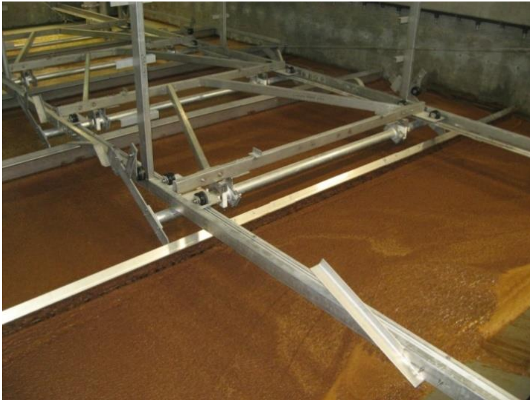
Figure 10. Penticton Water Treatment Dissolved Air Floatation
