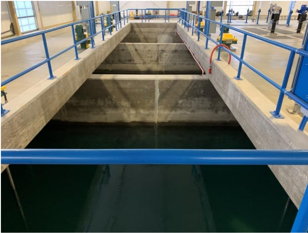
Figure 9. Penticton Water Treatment Floc Tank Mixers
