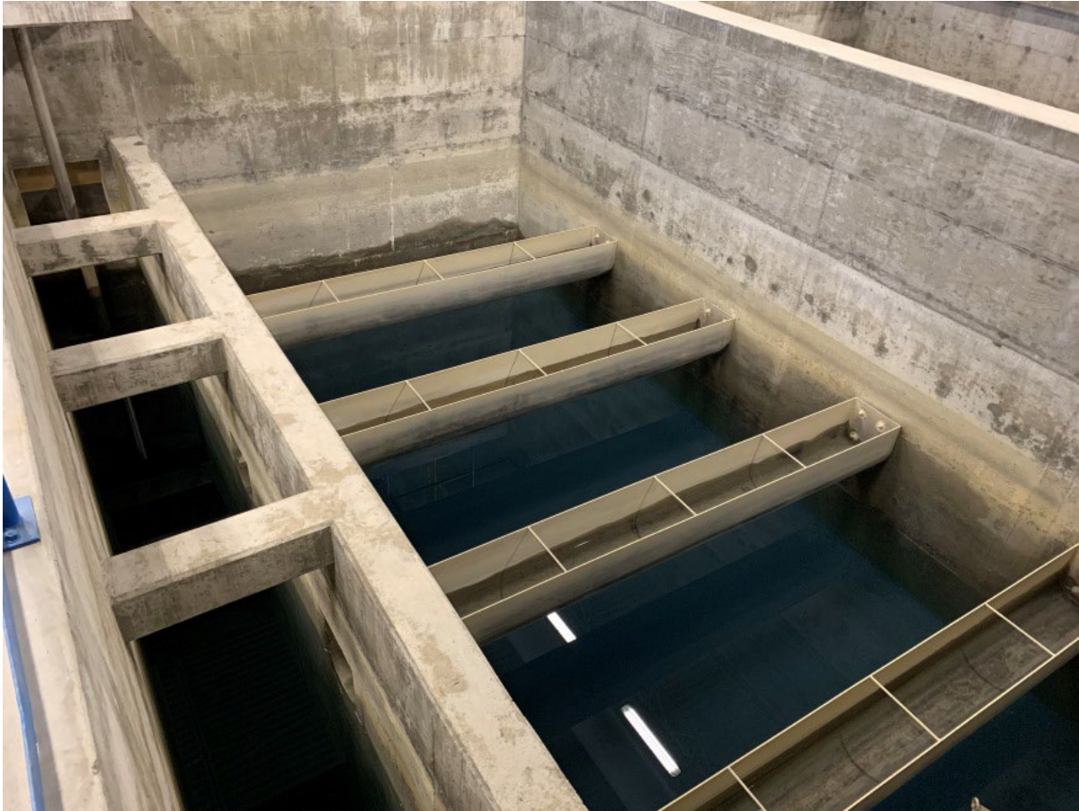
Figure 10. Penticton Water Treatment Mono Media Filters
