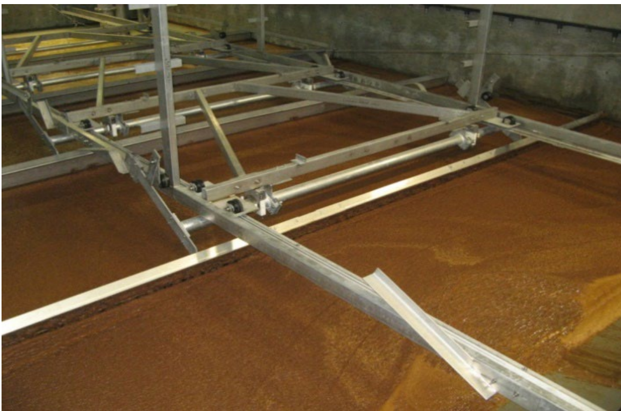
Figure 9. Penticton Water Treatment Dissolved Air Floatation
