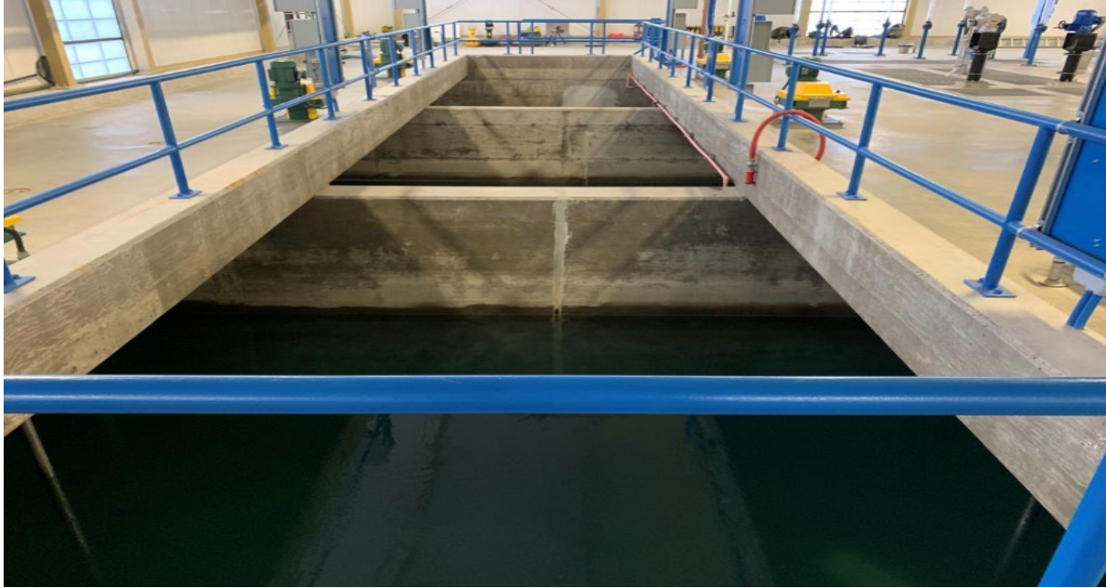
Figure 8. Penticton Water Treatment Floc Tank Mixers
