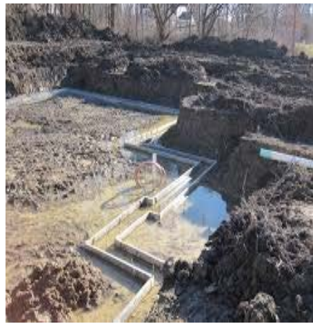
High Water in excavation
