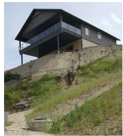
Steep slope development - erosion
