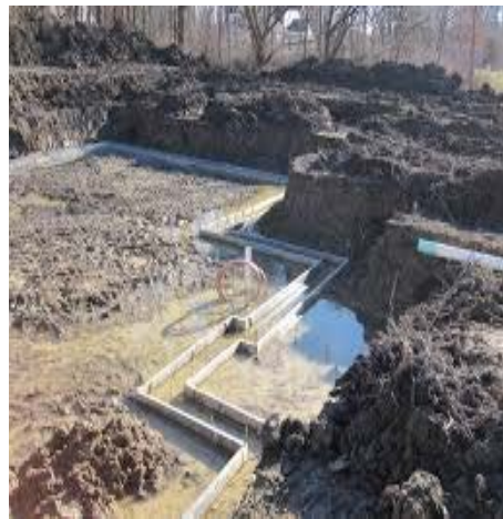
High Water in excavation
