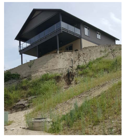
Steep slope development - erosion
