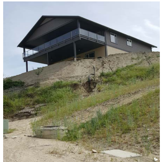
Hillside development – erosion issues
