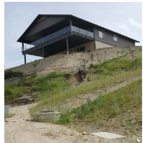
Hillside Development – Erosion Issues
