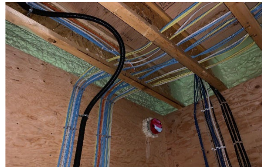
Mech. Rm - Unprotected foam plastics in joist spaces
