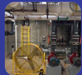
Use of a fan to ventilate space due to failed HVAC equipment
