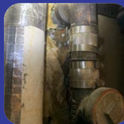
Mould growth due to failed sanitary line
