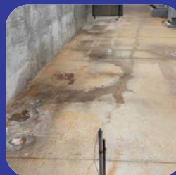
Ground water penetration due to failed perimeter drainage
