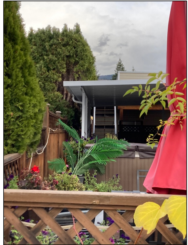
Figure 2 - Image of metal patio cover projecting on north side of the home.
