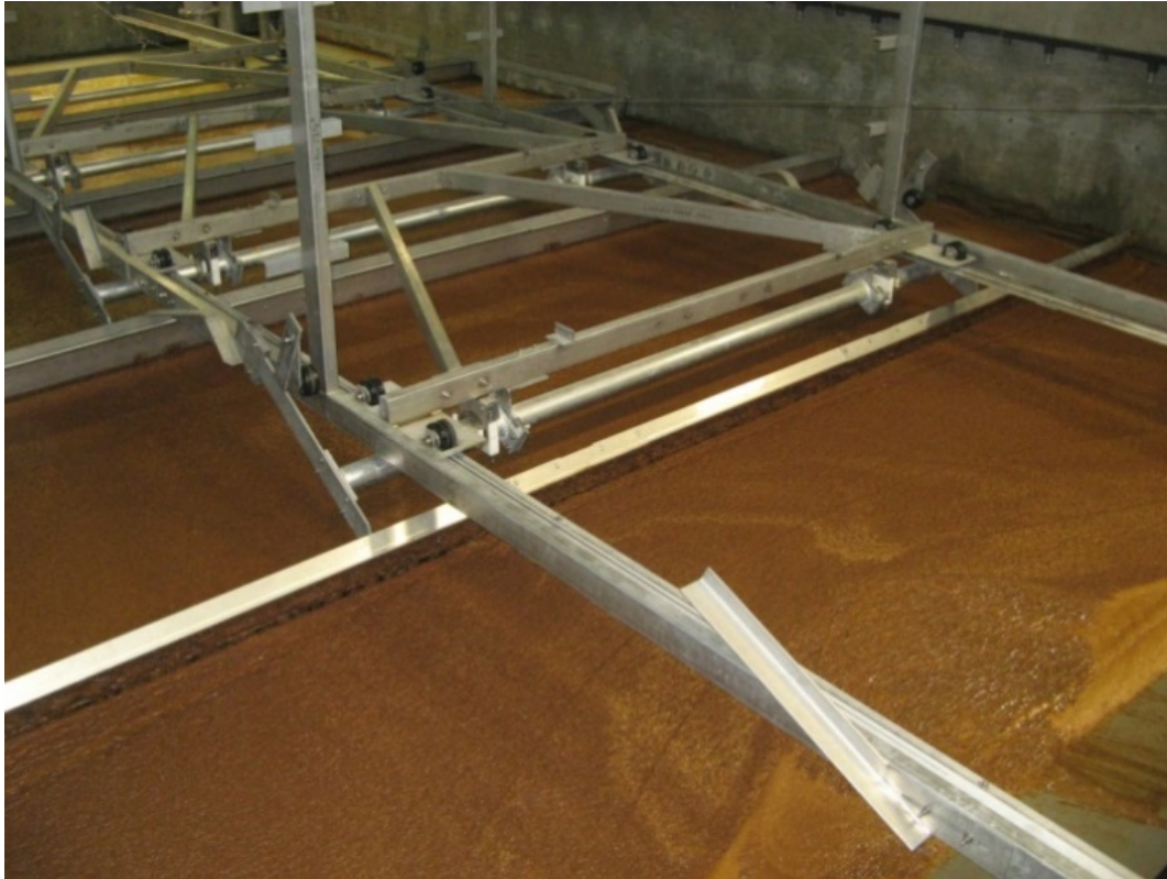
Figure 10: Penticton Water Treatment Dissolved Air Floatation
