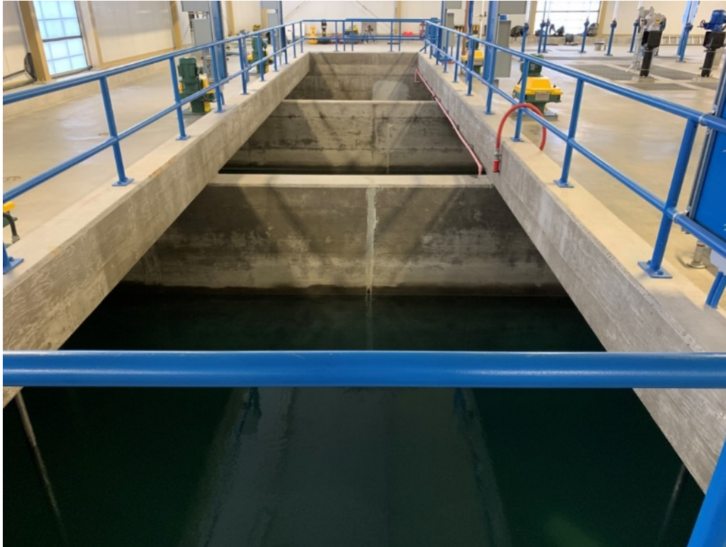
Figure 9: Penticton Water Treatment Floc Tank Mixers
