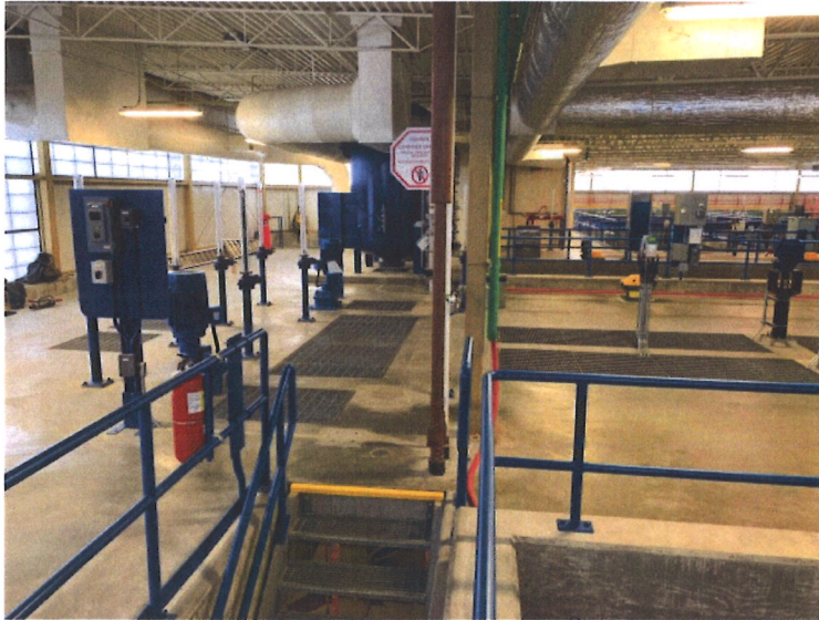
Figure 5: Water Treatment Plant Blend Chamber
