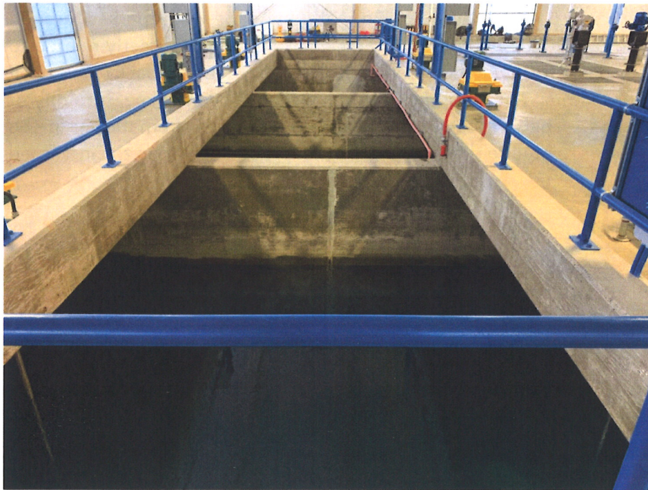
Figure 6: Flocculation Tank Mixers
