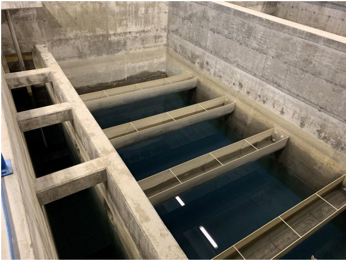
Figure 12: Penticton Water Treatment Media Filters
