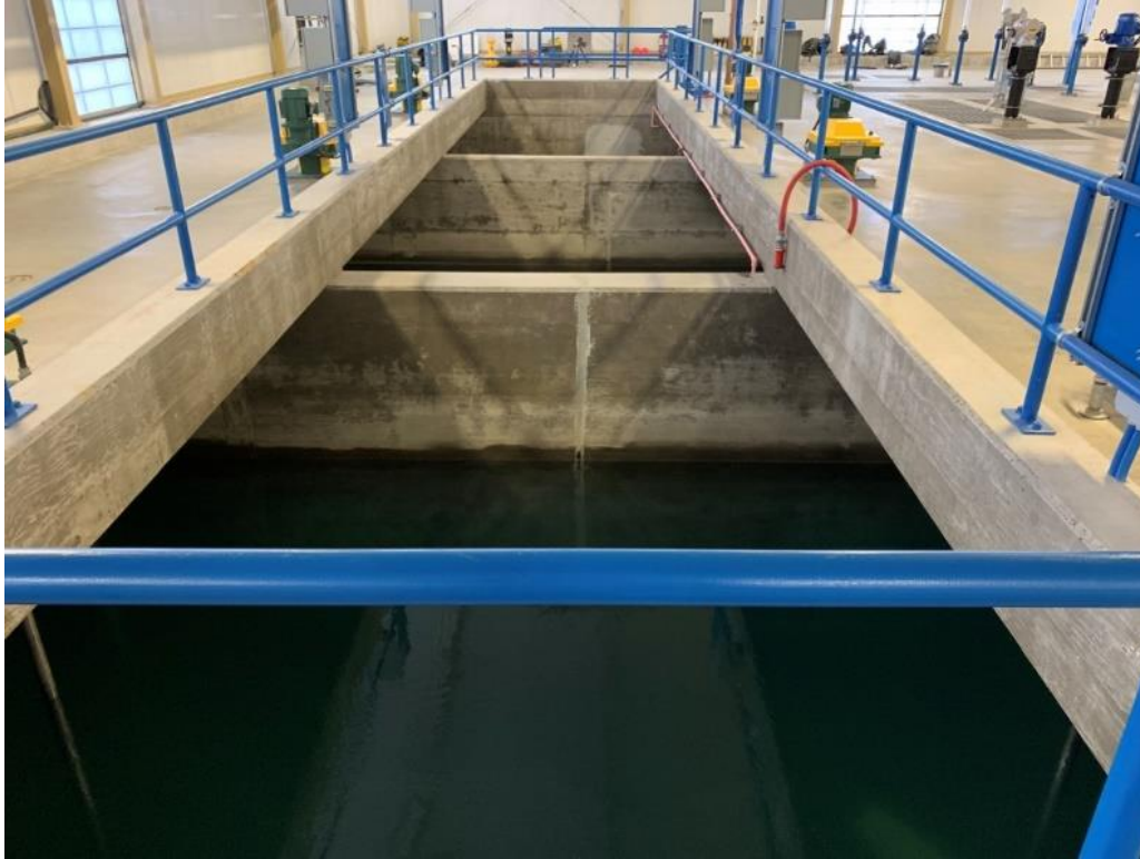
Figure 10: Penticton Water Treatment Floc Tank Mixers
