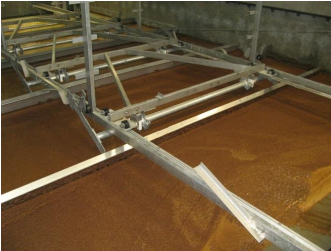
Figure 11: Penticton Water Treatment Dissolved Air Floatation
