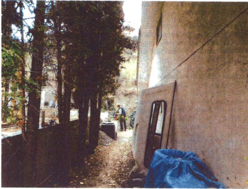
The photo below was taken on the April 3, 2014 shortly after the stop work order was taped to Ms. Laturmus' window. The photo shows the excavation, the dirt pile and the cut into the bank near the oversized retaining wall.
