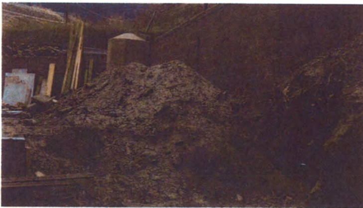
Nothing being done at 890 Three Mile Road will change this picture. 910 Three Mile Road will still be graded to drain onto Ms. Laturmus' property, there will still be a cut in
