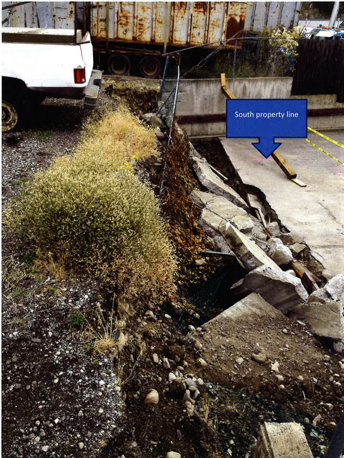
September, 2014 wall failure
