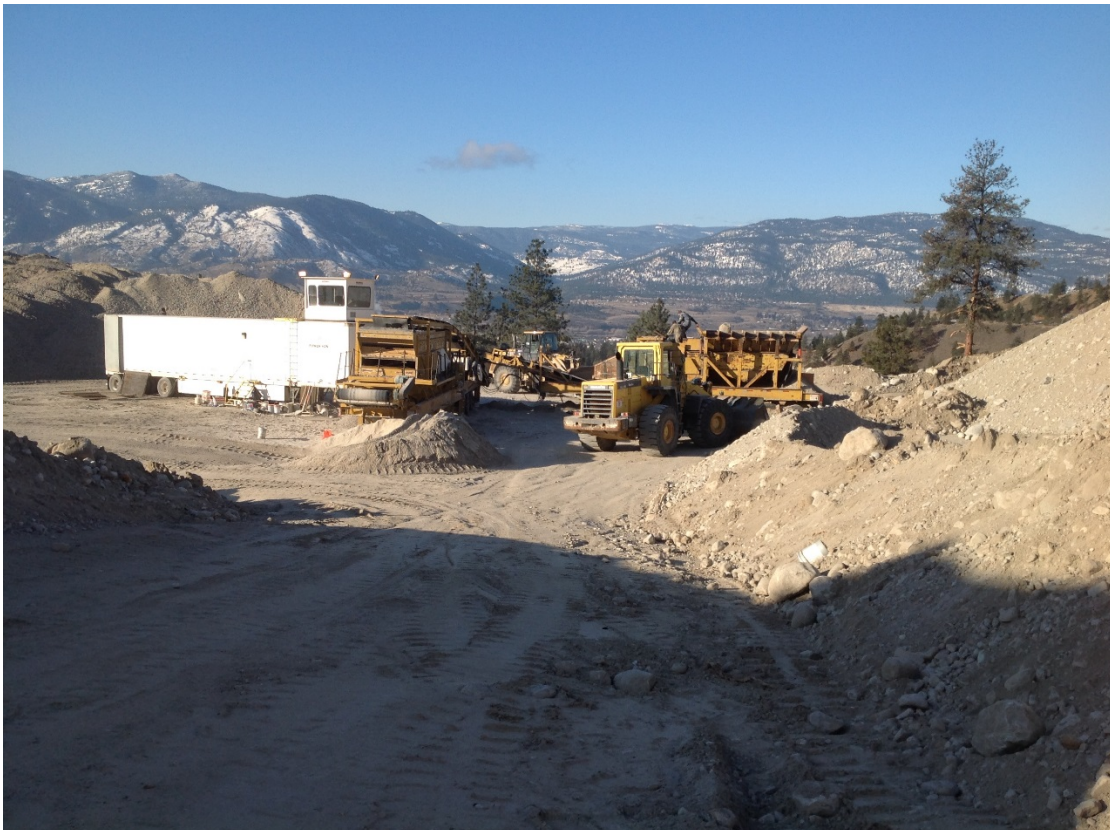
Figure 4: Image of crushing plant in place
