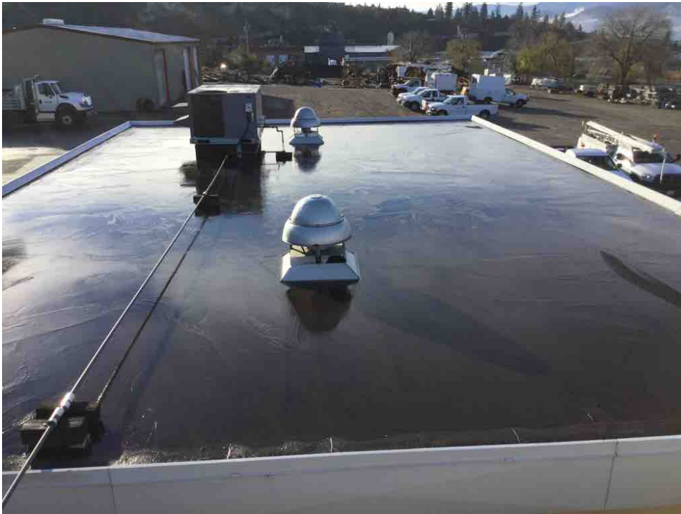
Significant ponding water noted.
