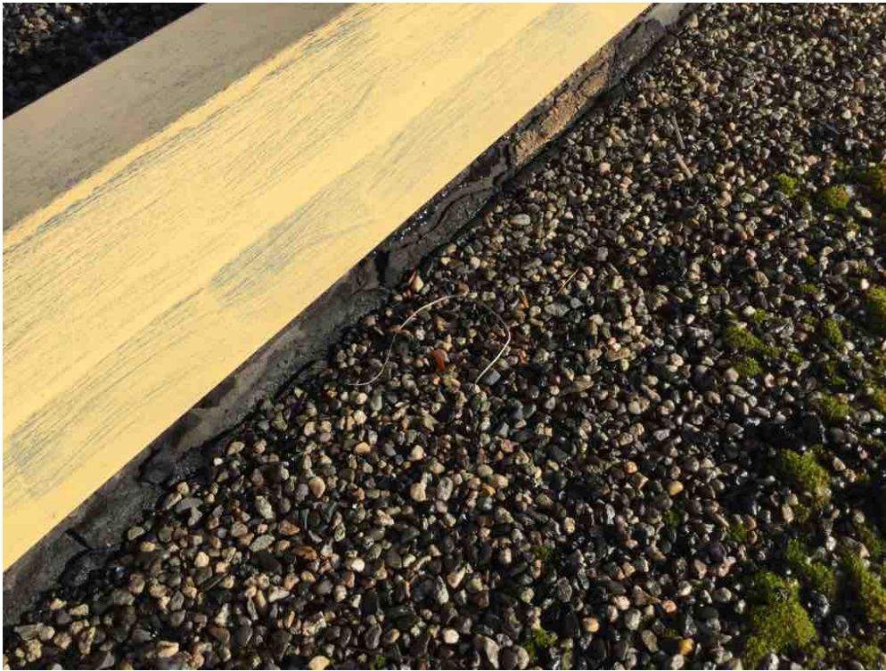
Roof membrane flashings are failing.
