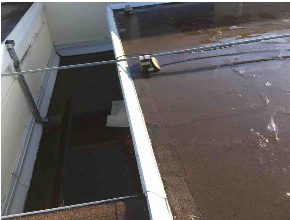
Metal cap flashing is in good shape with all joints sealed and securely fastened.
