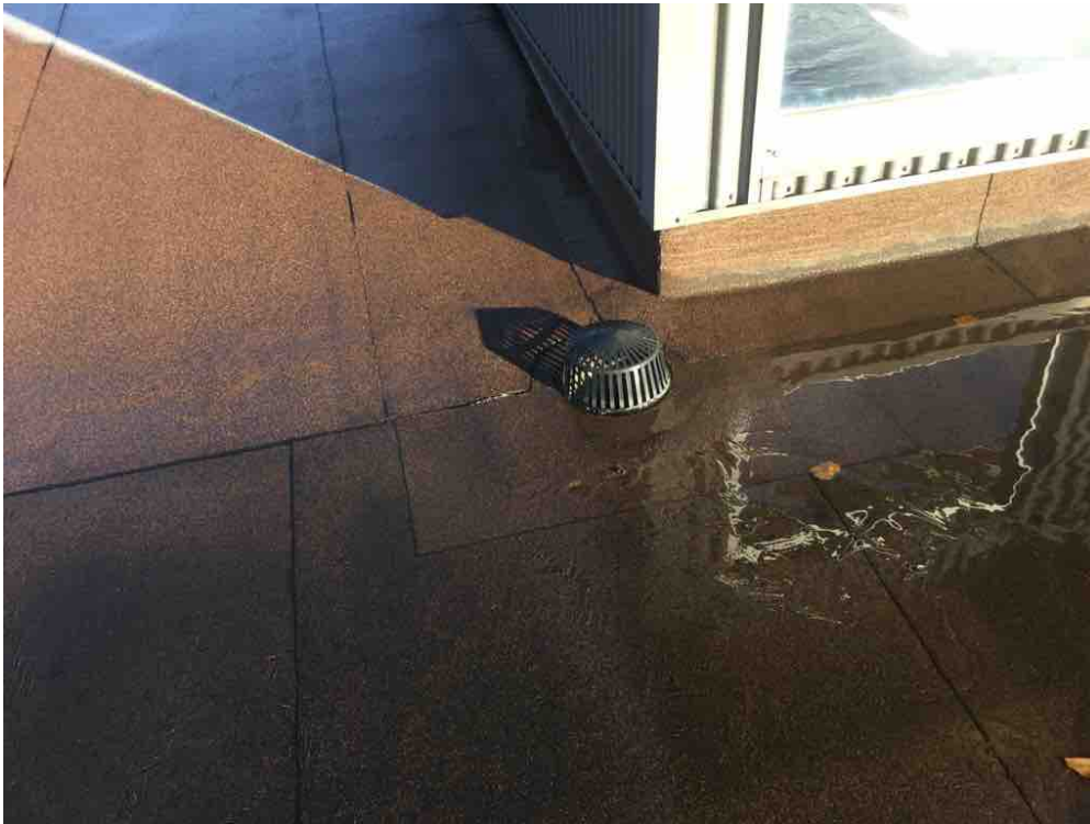
Drains are clear but insufficient slope to them does not allow the location to be effective.
