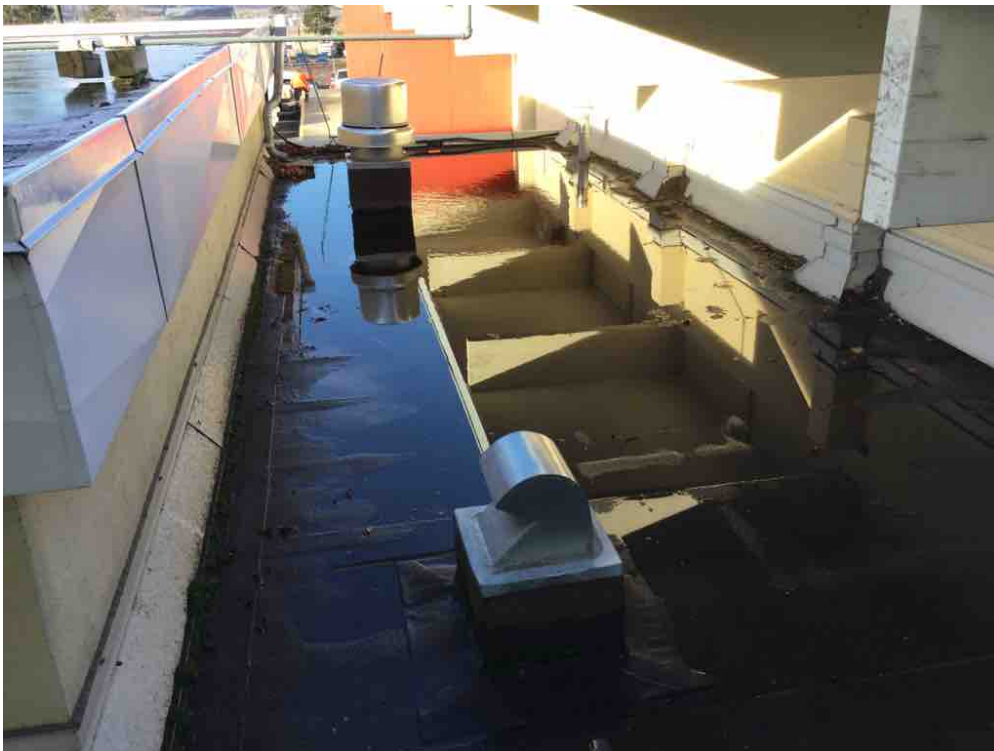
Significant ponding water noted.
