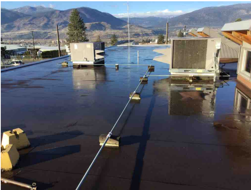
Flat portion of the roof has significant ponding water.
