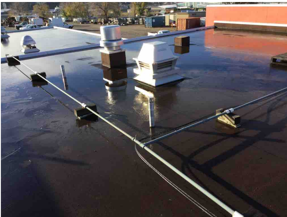
Significant ponding water noted.
