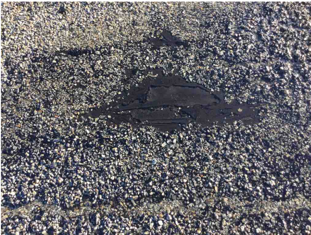
Degradation of the roofing felts on the exposed membrane is extensive.
