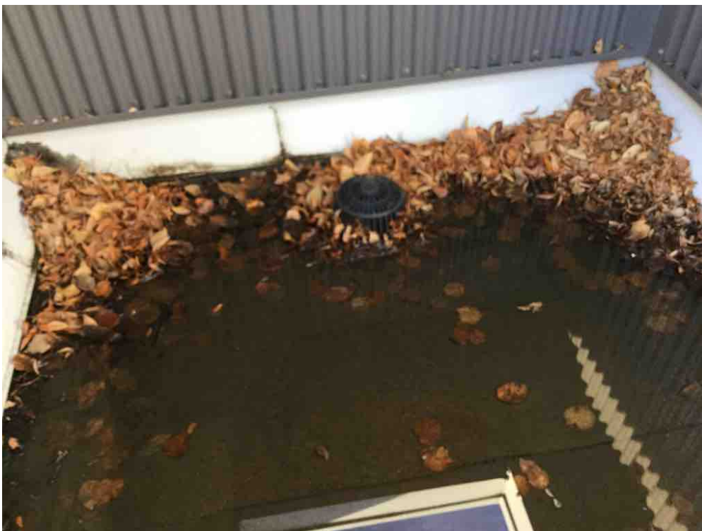
Debris is required to be kept away from drain in order for it to work effectively.
