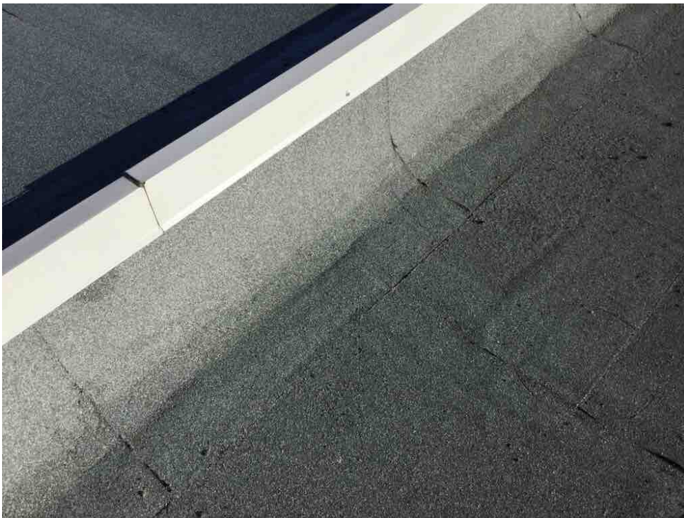
Wall stripping is well adhered.
