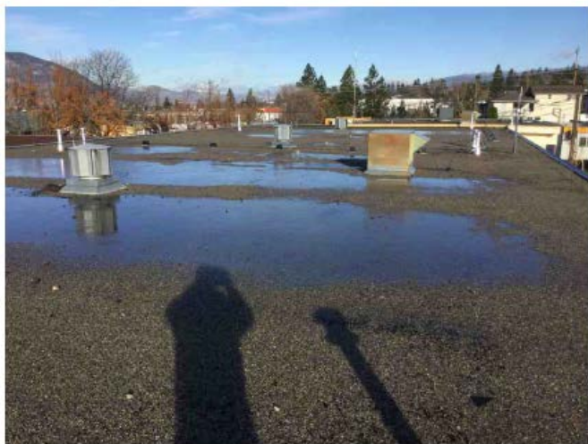
Figure 2. Water ponding on roof surface
