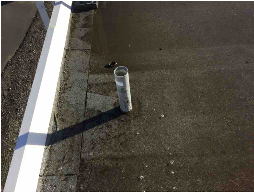
Settlement cap is missing.
