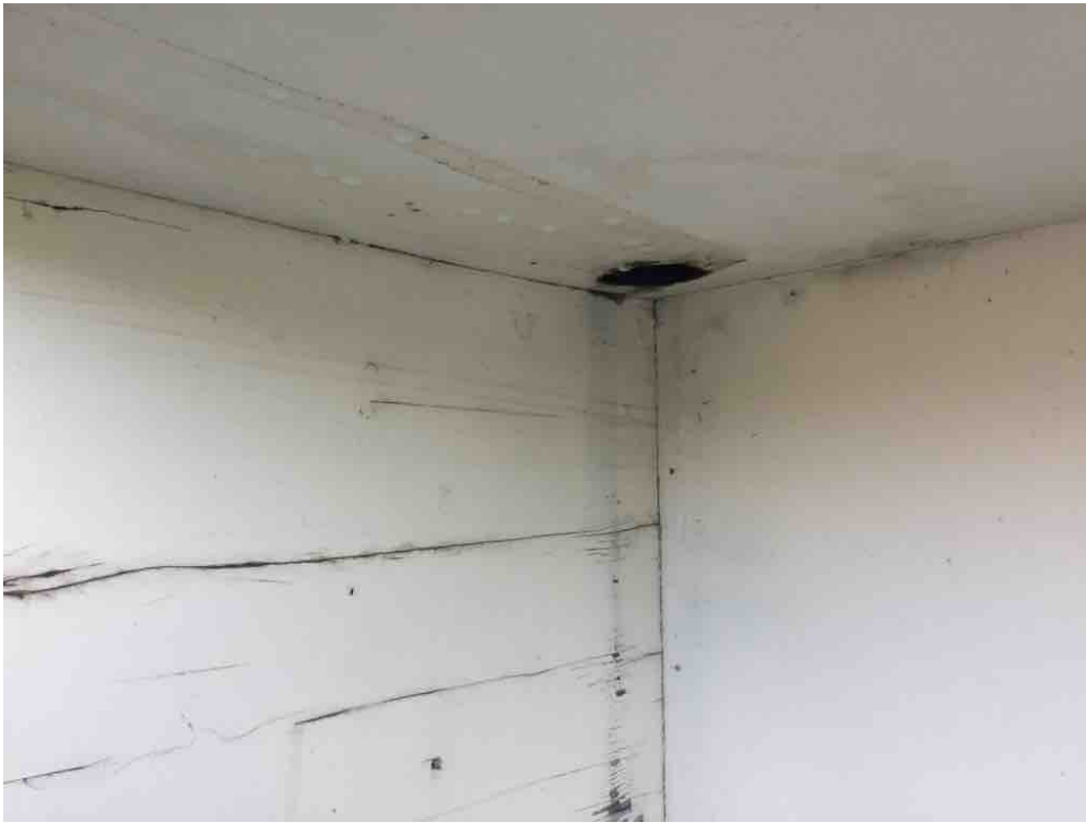
Downspout is missing and water is now running along the soffit.
