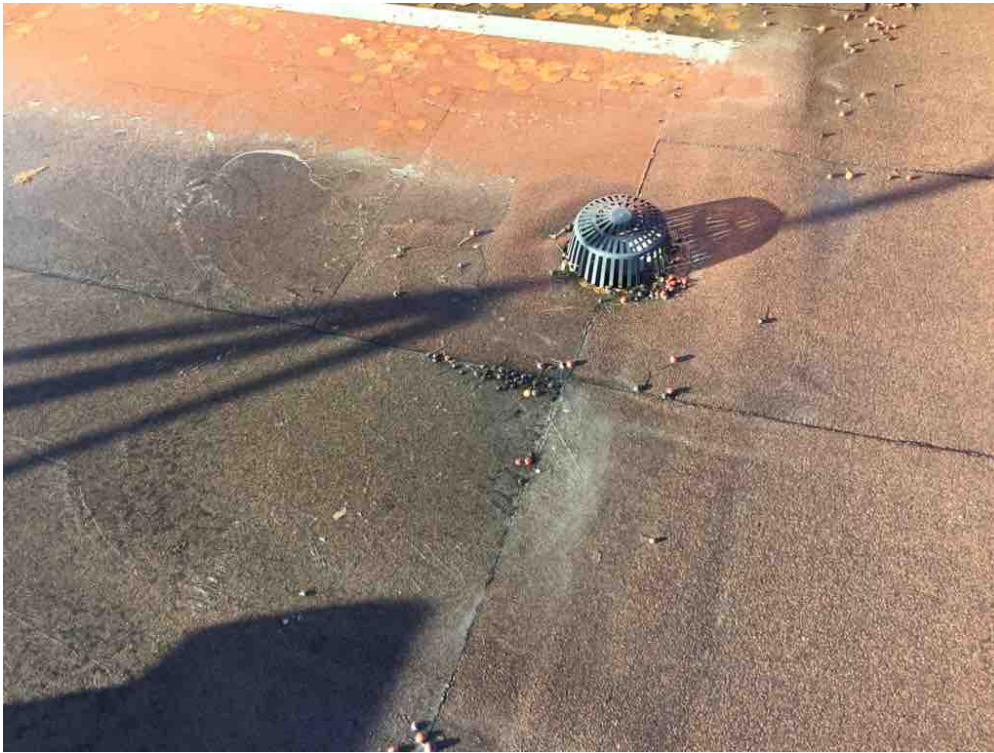
Drains are clear but are located at the high point of the roof.
