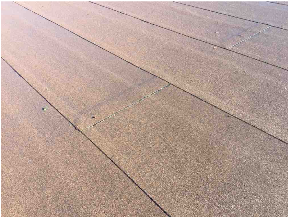
The roof membrane is in excellent condition but several blisters have formed that require attention.
