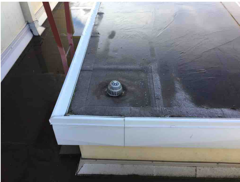
Drain location is dry.
