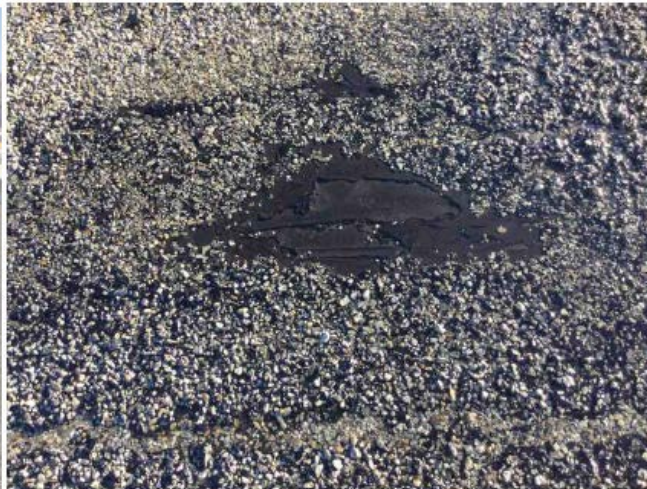
Figure 3. Degradation of roofing felts and membrane
