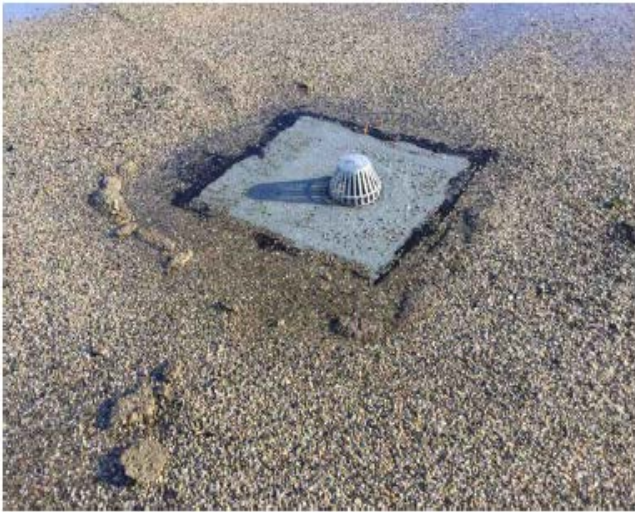
Figure 4. Compromised roof felts and membrane
