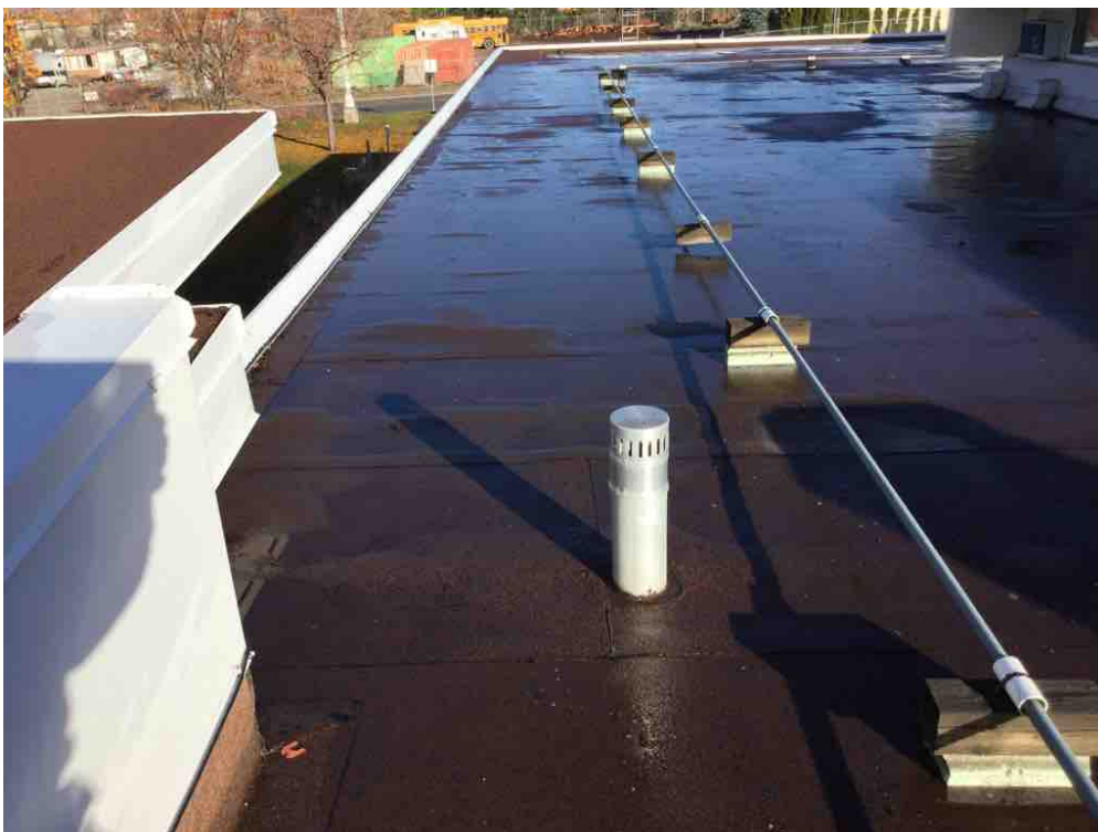
All blisters should be repaired.
