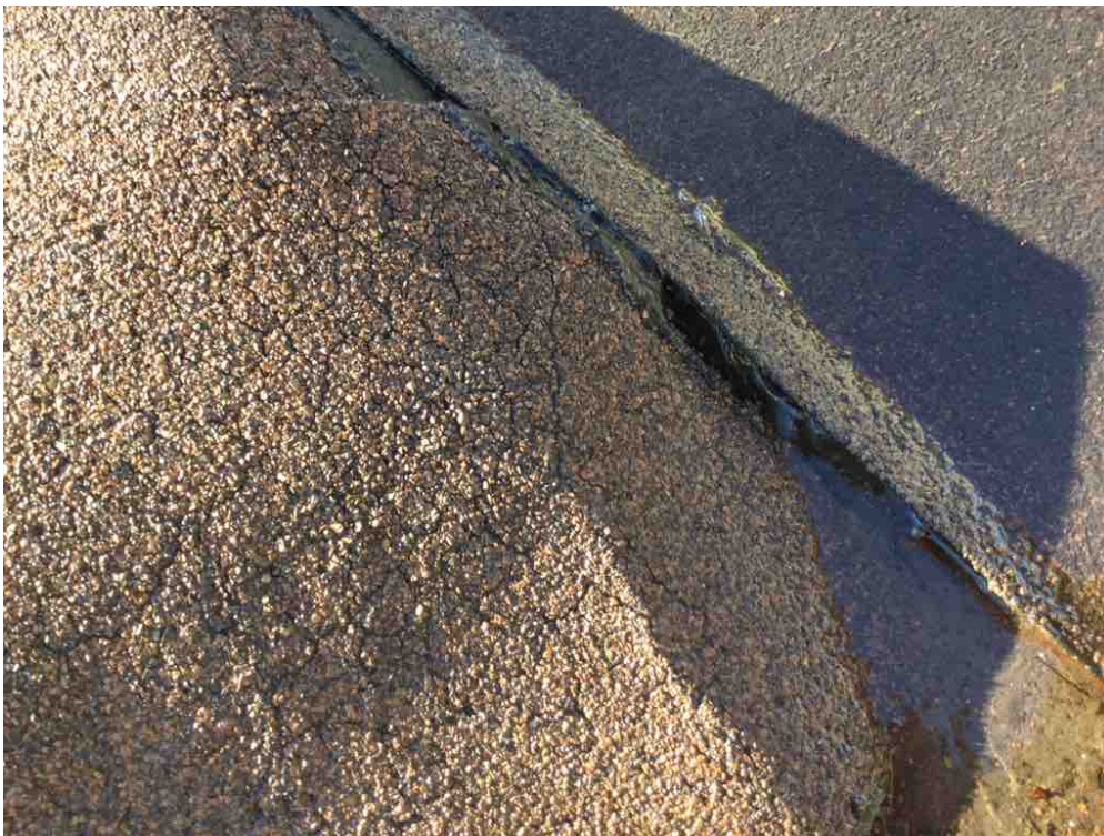
Open seam is allowing water to migrate between the ply's.
