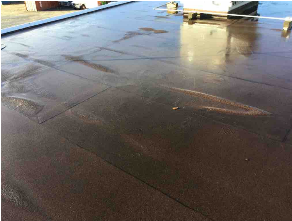
Blistering prevalent throughout.
