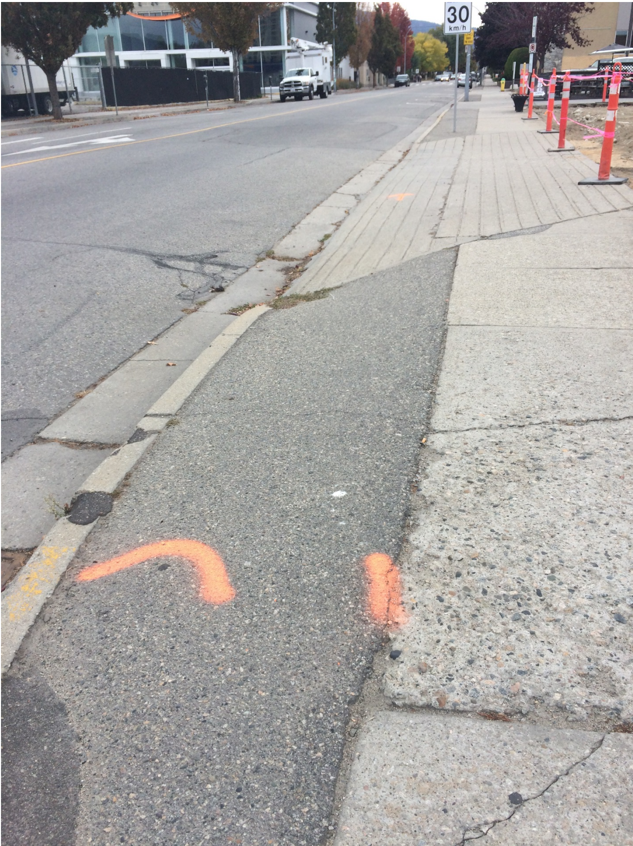
Figure 3: Image showing the condition of the sidewalk and frontage at the corner of Westminster Avenue and Winnipeg Street, looking down Winnipeg Street
