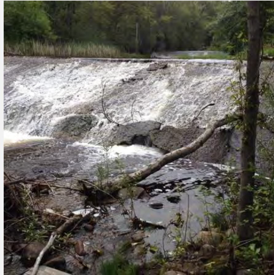
Water flowing under the concrete apron of Structure #36
