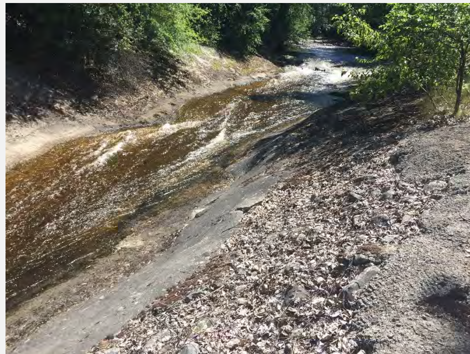
A concrete lining hole with visible mesh
