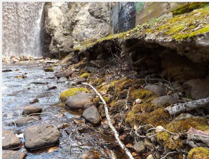
Evidence of Creek Downgrading Below Penticton Dam #2
