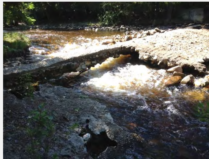
A failed concrete structure in Reach 9
