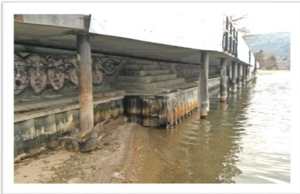
Area beneath pile supported walkway showing gap under the slab.
