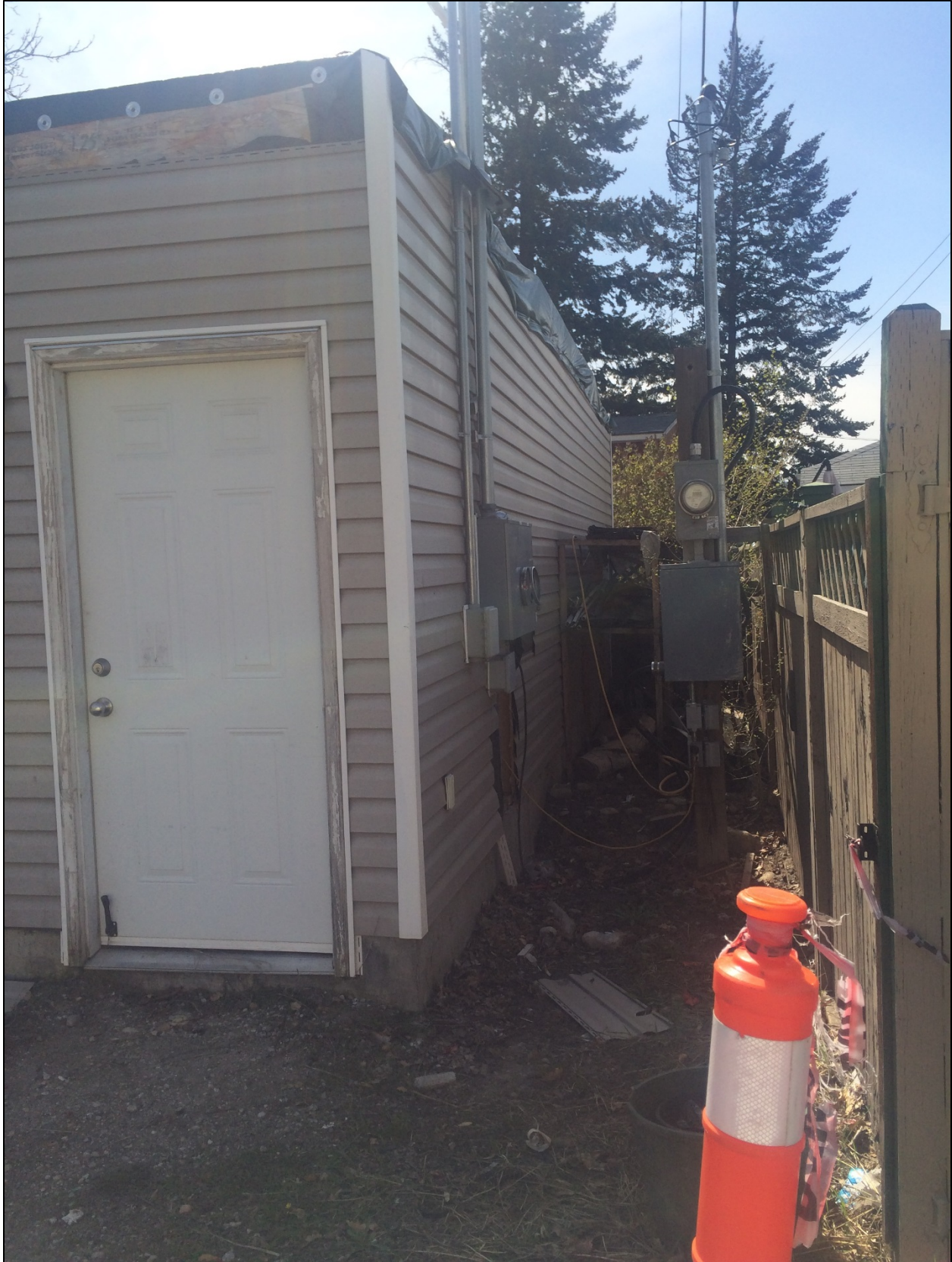
Figure 6 – Looking down northern property line of side yard at 920 Kilwinning Street (variance requested)
