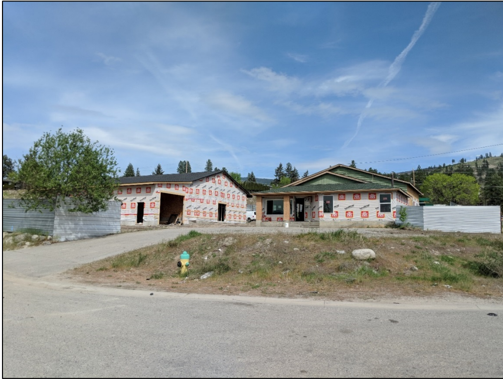
Figure 5: West View of Existing Buildings currently under renovation on Proposed Lot A (from Commercial Way)
