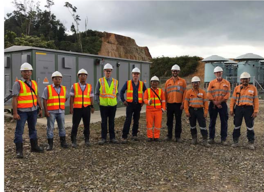
Photo: StruthersTech Representatives from Indonesia's state-owned power utility PLN, StruthersTech Engineers and PT Agincourt mining personnel pose in front of the power compensation equipment upon successful commissioning.
