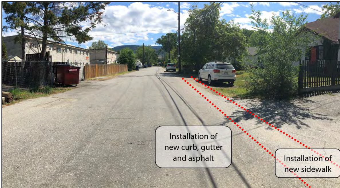
Figure 6 - Looking east along Churchill Avenue, which will receive new asphalt, curb, gutter and sidewalk on the south side of street
