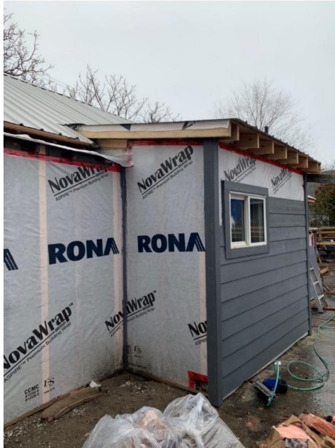
A photograph of the exterior of the bathroom group that was added without a review and in a section of the single-family dwelling that may not have a foundation.
