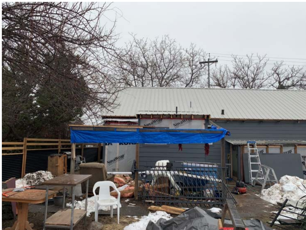
A photograph of the low slope roof section that had metal roofing, which is not permitted by the British Columbia Building Code.
