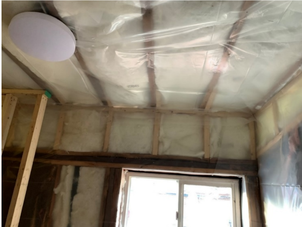
A third photograph of the interior of the bathroom group that shows the insulation of the exterior walls and in the ceiling of the low sloped roof. The insulation of the room was required meet the values given in the British Columbia Building Code and to be noted on the revised drawings.
