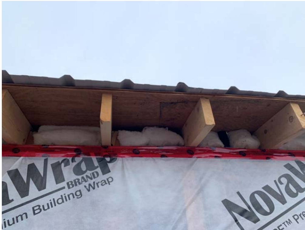
A close-up photograph of the low slope roof of the bathroom group that is unvented, but is required to have vents by the British Columbia Building Code.
