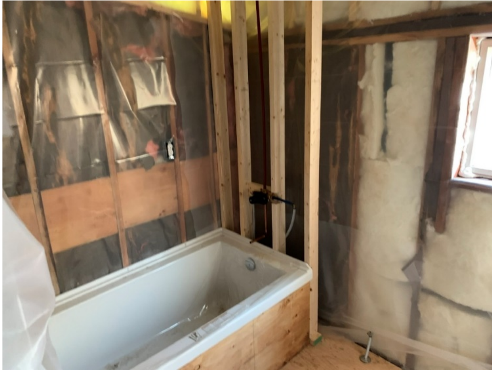
A photograph of the interior of the bathroom group that was not included in the drawings that were submitted for the building permit BP012918. One of non-compliant issues with this room is that the exterior walls are not constructed of full studs which results in a 'hinged wall'.
