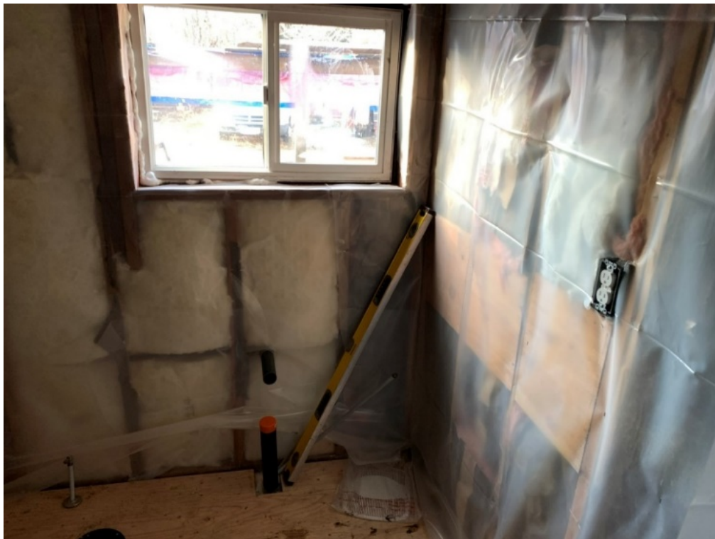
A second photograph of the interior of the bathroom group that contains a window that lacks a required lintel.
