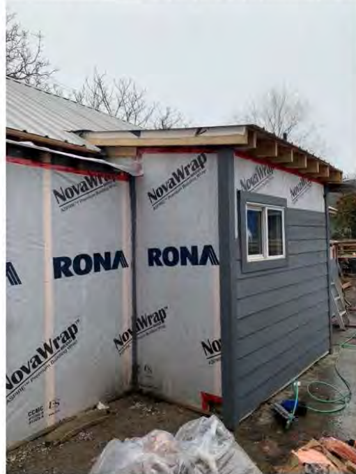
A photograph of the exterior of the bathroom group that was added without a review and in a section of the single-family dwelling that may not have a foundation.
