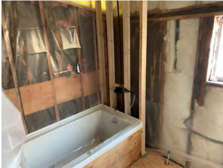
A photograph of the interior of the bathroom group that was not included in the drawings that were submitted for the building permit BPO12918. One of non-compliant issues with this room is that the exterior walls are not constructed of full studs which results in a 'hinged wall'.
