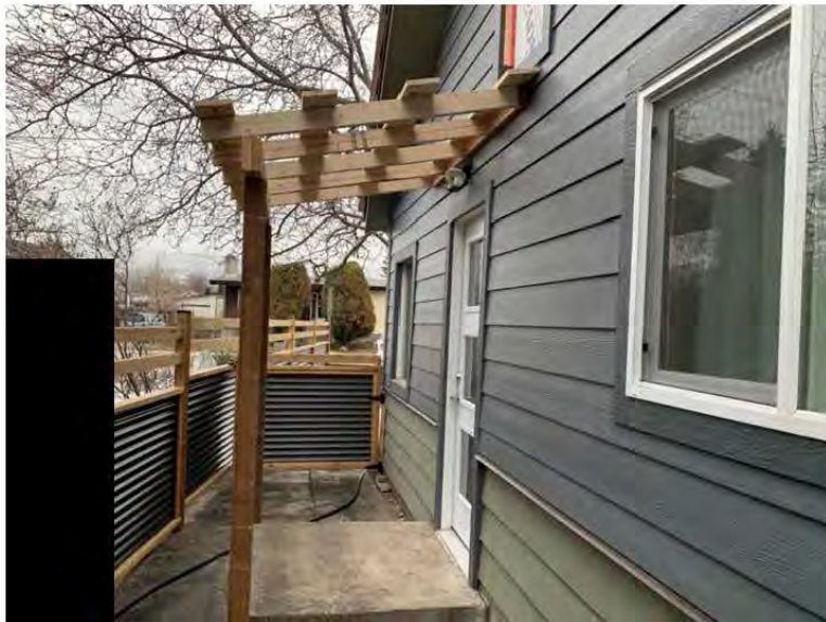
A photograph of an unpermitted addition of a covered entry on the north side of the single-family dwelling at the Property. The noted deficiencies for the covered entry include the 4-inch by 4-inch posts and a ledger that has been improperly attached to the exterior wall through the new siding.
